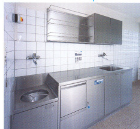
| Contaminated sluce room after modernisation.
